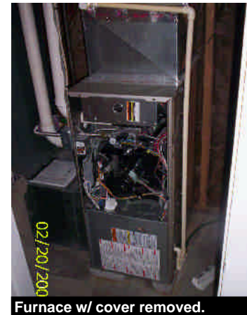
Furnace w/ cover removed.
