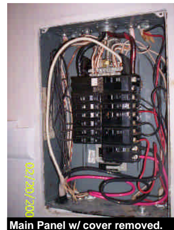
Main Panel w/ cover removed.
