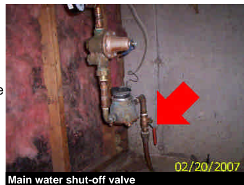
Main water shut-off valve
