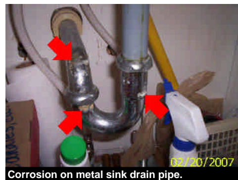
Corrosion on metal sink drain pipe.
